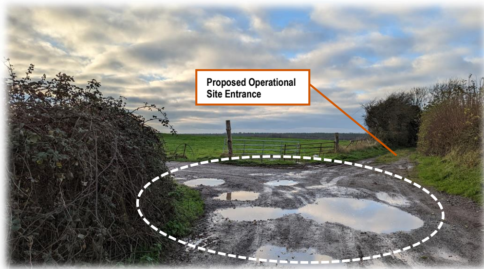
Figure 2.4 – Existing Failed Pavement
